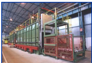
Continuous T6 Heat Treat
